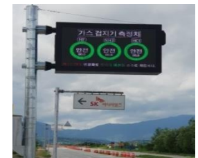
[Gas Gauge Display Board]
